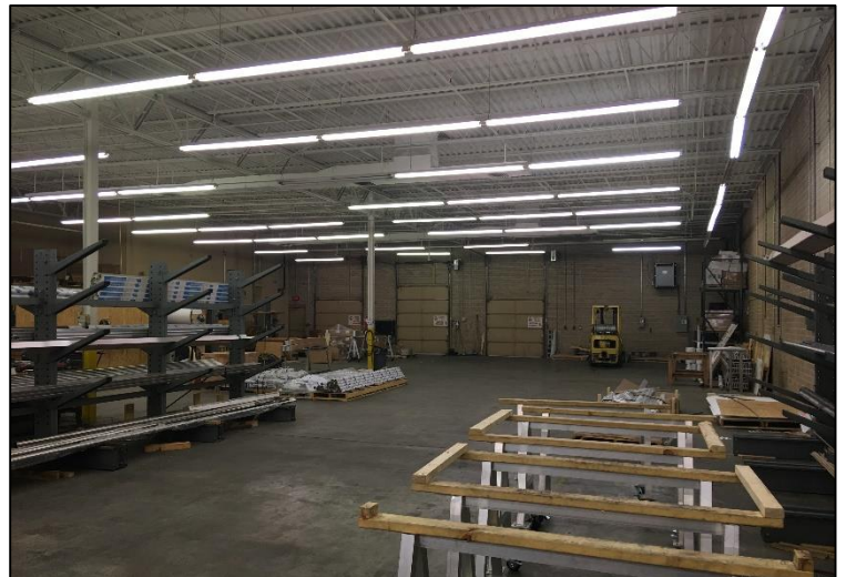
HVAC In the Warehouse
